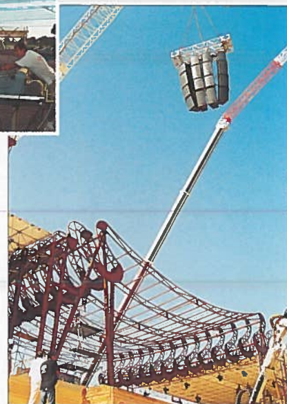
Top, the main cluster being moved into position. Marcello Notari (left) with Utilas site manager Di Rienzo after set-up
